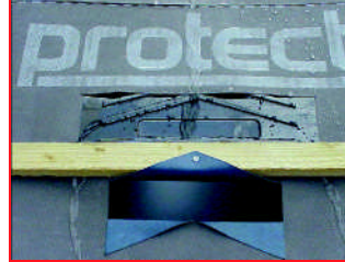
~ An L shaped component resting against the batten and slotted through a slit in the underlay diverts the water running down the underlay around the correctly sized rectangular hole. Pulling the underlay up and nailing it to the batten assists the water to flow away from the hole. (Photo courtesy Building Product Design Group)
