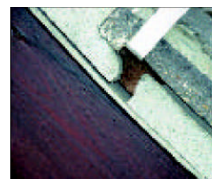
~ It is possible to clearly see the end of the batten through the crack in the mortar bedding, an ideal entry point for water.
