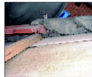
~ Poor detail – the end of the batten is embedded in the mortar, causing the mortar to crack at each batten position,
