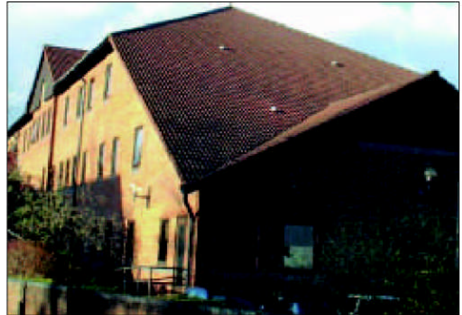
- The choice of a bold roll interlocking tile on such a long rafter length is excellent. But collecting all the rainwater run off into a valley and expecting a small hopperhead and down pipe at the bottom of the valley to cope with the high volume of water, is not.
