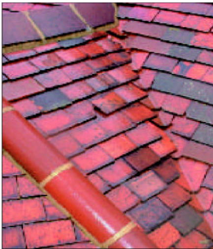
- The rafter pitch on the left is 35° and the pitch on the right is 50°. Both were set out at 100mm gauge. Note how many courses there are on the left compared with the right. An open lead valley should have been formed between the two slopes.
