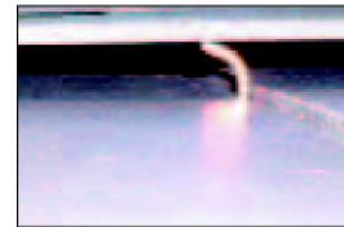
~ Unless the tail rivet is bent at right angles, the upper slate can pull off the copper disc rivet pin under high wind uplift loads and then sit on the head of the pin.
