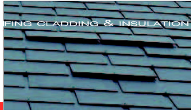
~ Fibre cement slates that have pulled off the copper tail rivet pins will sit on the head of the pin producing a 15mm gap up through which wind and rain can drive.
