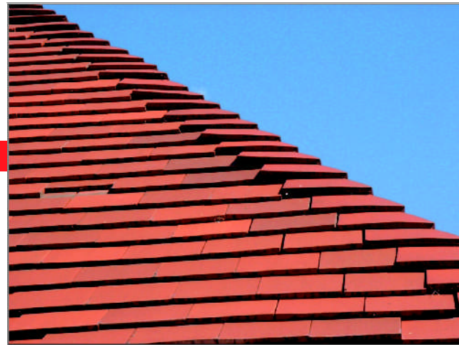
- The clay arris hip tiles on this roof were not sorted correctly. While some of the hip tiles fit correctly, others kick out badly. Note how tile and a half's have been used to maintain the half bond.
