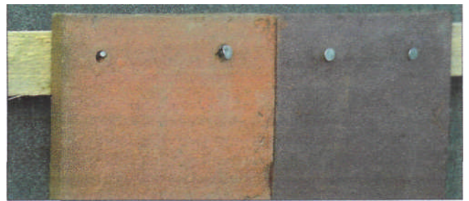
• The heads of 40 by 2.65mm aluminium clout head nails are very thin. Under high wind suction the left hand nail head has pulled off, the middle nail head has started to fold up and the right hand nail is new, but just as thin.
