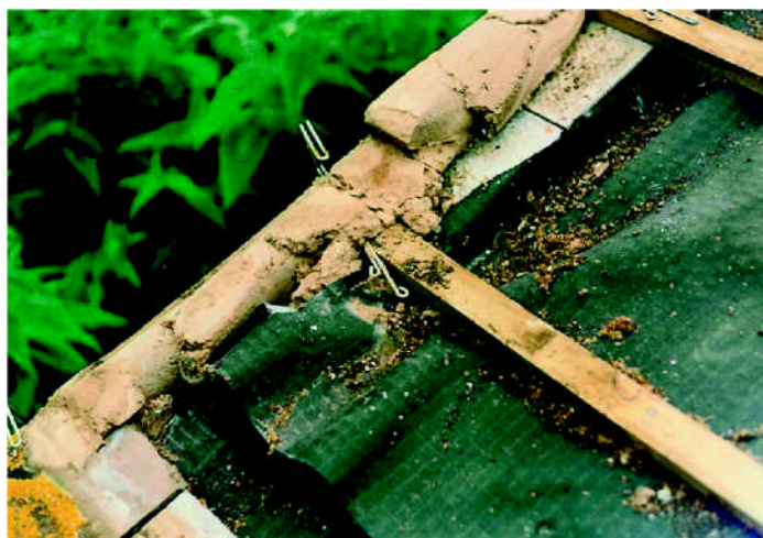
There is nothing right about this verge. The verge clip is not nailed to the batten, the battens finish in the mortar, and the underlay is laid above the undercloak and sinking down into the cavity wal.
