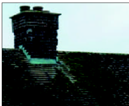
limited area of roof free from moss.
