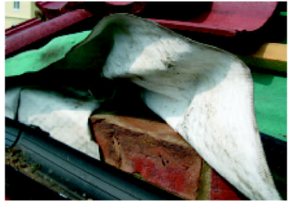
The top of the brick wall was just right for the single pantiles, but the VP underlay was draped behind the gutter with no underlay support board. The eaves comb was not nailed to the top of the brickwork allowing birds to nest in the batten cavity, the guttering was screwed into a brick joint and set too low for the tiling, and the eaves tiles were not nailed or clipped
